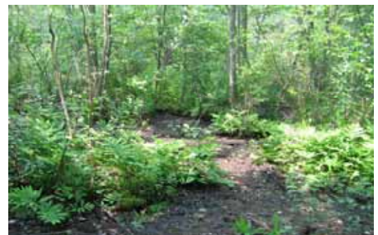
This wetland area off Hope Street and was scheduled for remediation. NEE delineated the resource areas and designed the wetland restoration plan. Approximately 16,860 square feet of wetland soil will be removed and restored followed by the installation of native wetland plants.
