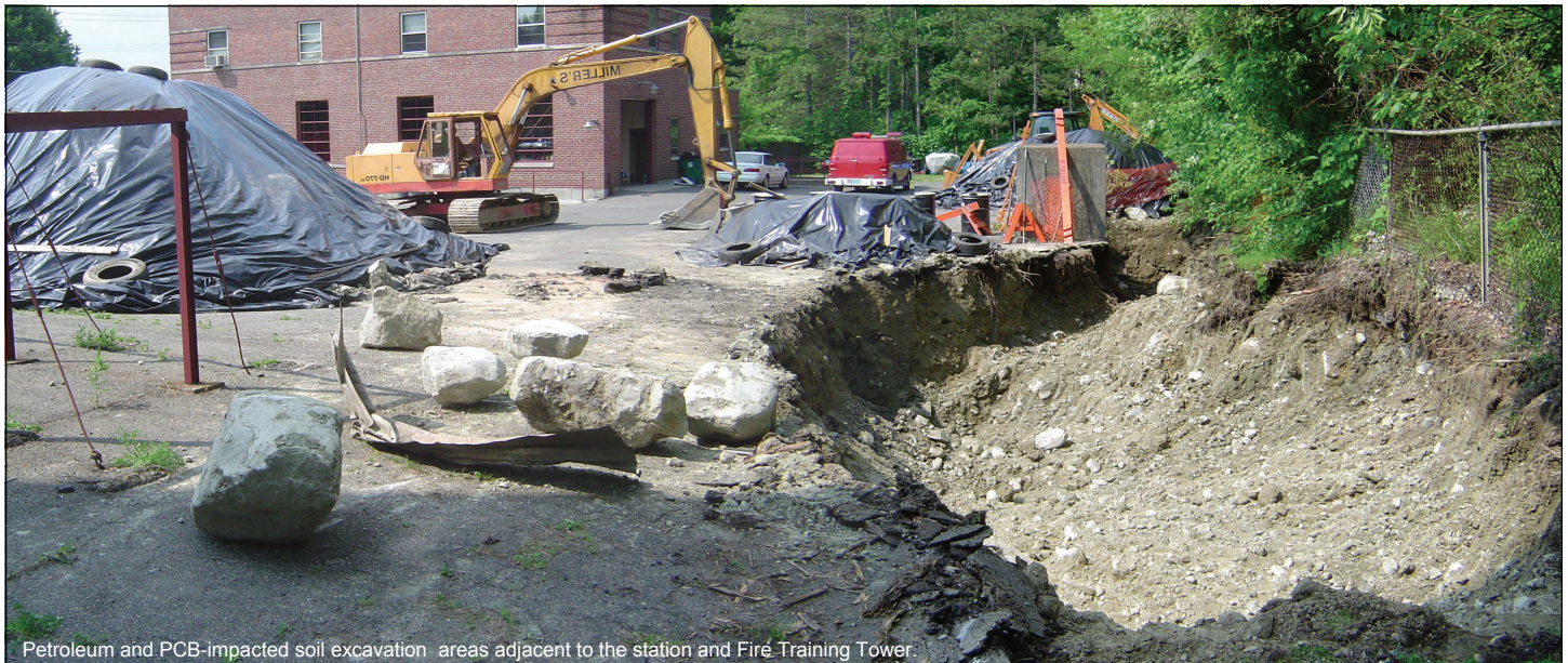
Petroleum and PCB-impacted soil excavation areas adjacent to the station and Fire Training Tower.
