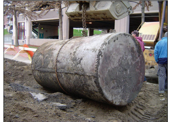
A 54-inch by 8'-8" riveted steel #2 fuel oil underground storage tank being removed.
