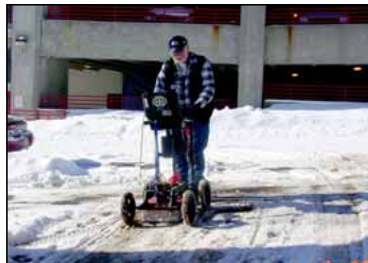
Ground Penetrating Radar (GPR) was used to locate historic underground storage tanks and current utilities prior to drilling.
