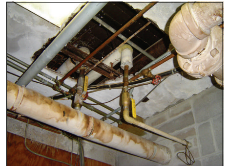
Confirmed asbestos-containing pipe insulation.
