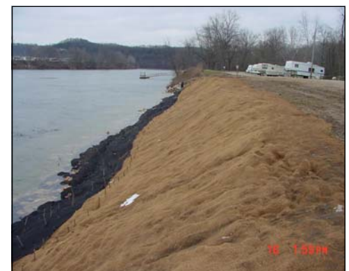
Re-graded bank with permanent erosion control fabric and biodegradable erosion control blanket along the slope.
