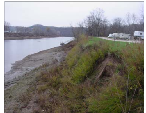
Eroded bank prior to site excavation.
