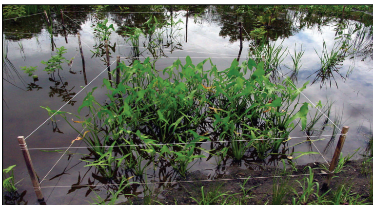
NEE installed native wetland plants, including Sagittaria latifolia , within the isolated pond. Temporary wildlife fencing was placed around each aquatic plant bed to prevent predation by waterfowl until the plants were fully rooted.
