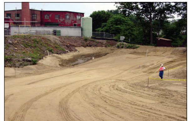
Condition of the isolate pond area following excavation of impacted soil and re-grading.
